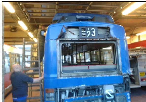
Volunteers rebuilt the rear of Leyland National Mk 1 to repair or replace corroded panels prior to repainting in its original colours as Leyland test bus REV01
